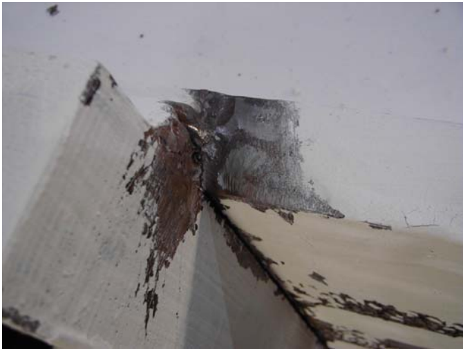
Figure 14. At 3\delta_y a crack at the tip of the beam flange at the termination of cover plate was observed in all three specimens. This crack however did not grow in size or length during the remaining cycles of the test and did not adversely affect the hysteretic characteristics.
