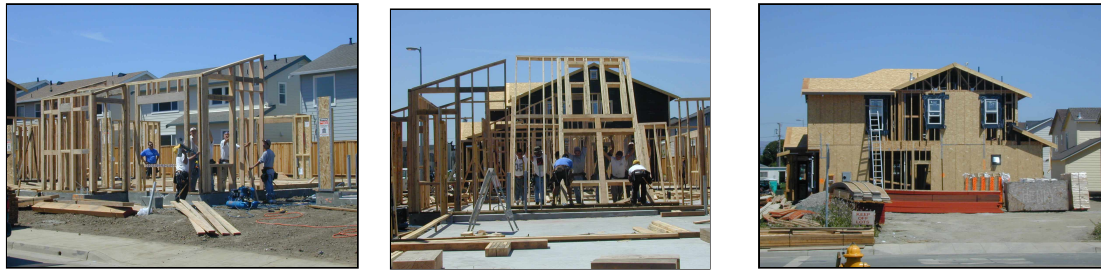
Figure 4: Illustration of Construction Process for Wood Frame Construction in the U.S.A. (Arnold [17])
